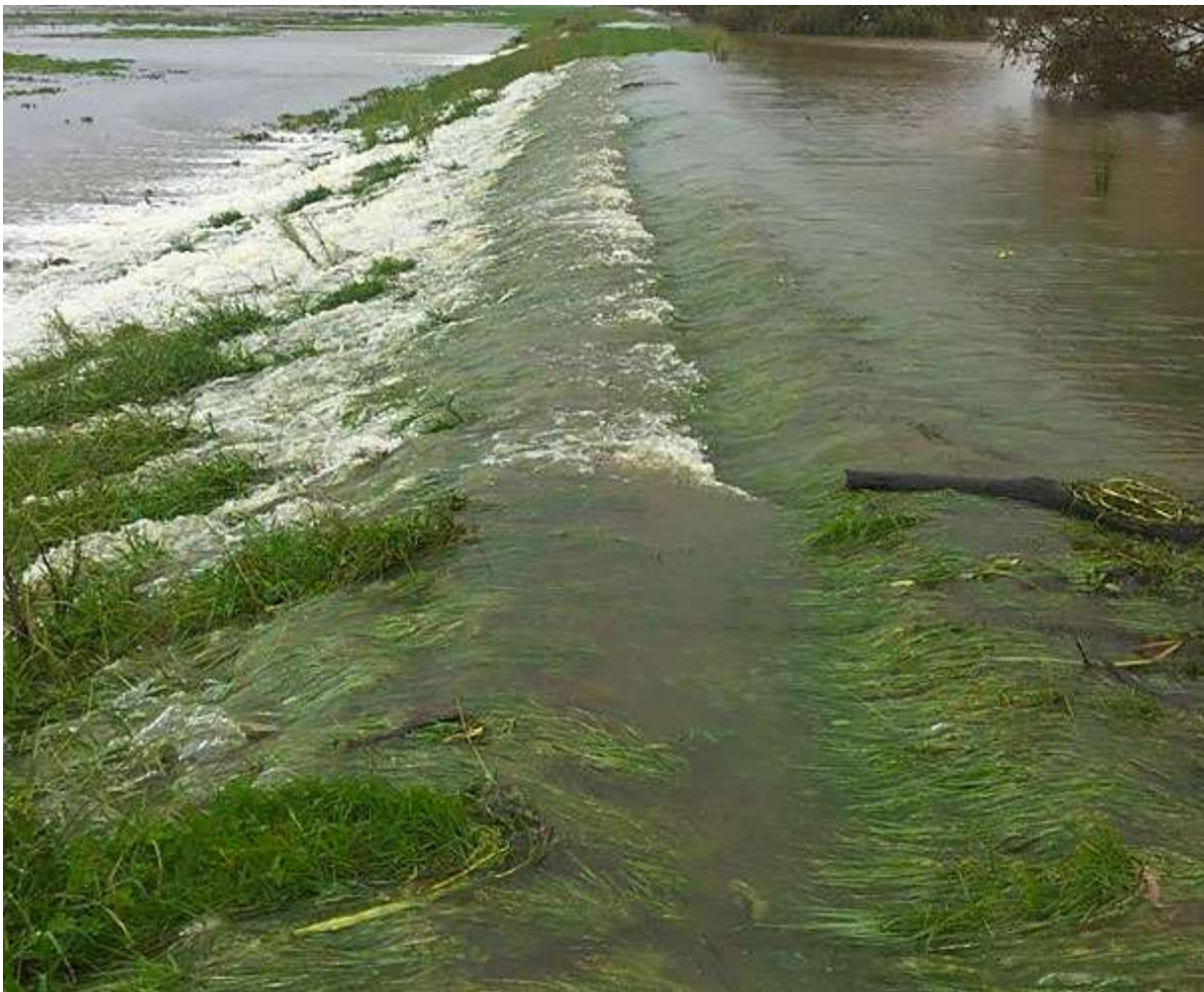
Overtopping of the stop-banks and inundation of Hauraki Plains by the Piako River flood in April 2017 (NB This 100-year flood event far exceeded the 50-year flood-event design capacity of the existing scheme).
