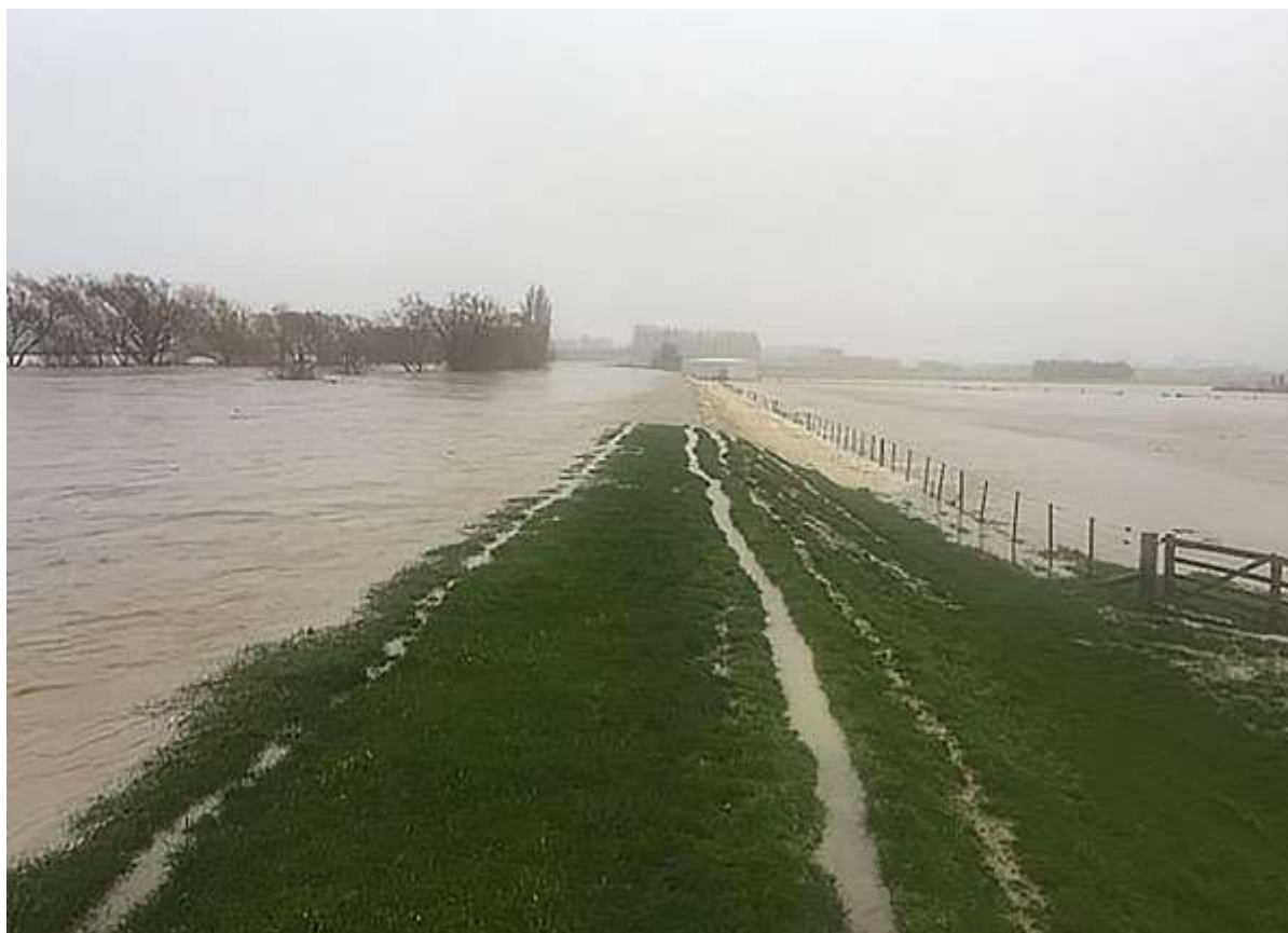
Photo: Selwyn River stop-bank overtopping in July 2017.
