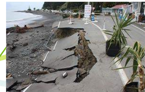
Erosion at Clifton
